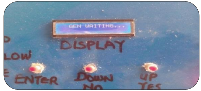
Fig 8: Display during generator stabilization
