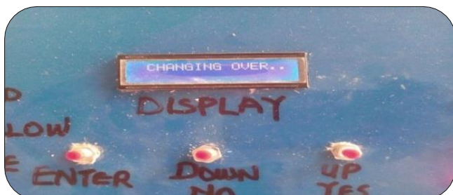
Fig 7: Display during changeover from public utility to generator
